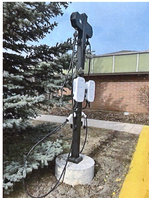
Level 2 charger at School Board Office
